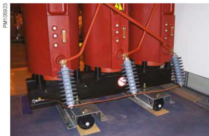
High voltage surge arresters on the lower part
